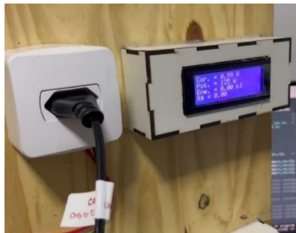
Figure 10 - Image of the wooden panel and the power box (left), as well as the display. LCD to display real-time readings (right).
